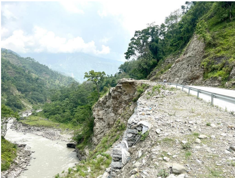
Damaged Road Section along Barhabise-Bhotekoshi Municipality Road Section
