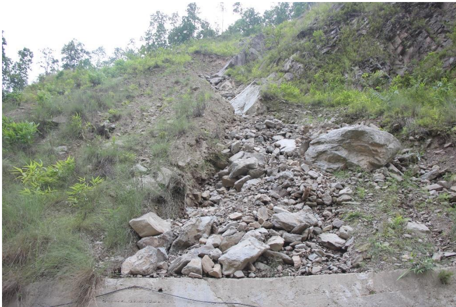
Rock fall at Balefi Rural Municipality Ward no 1
